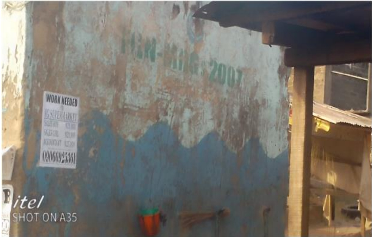
Fig 5. Abandoned MDGs water project, Oke-Ori Omi, Ado Ekiti.
