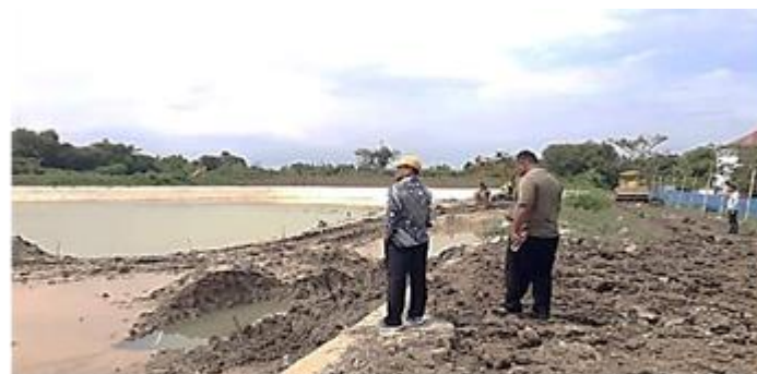
Drainage Detention Basin FMNJP in Padakaton Village, Cisanggarung River area, Brebes Regency, Central Java Province
