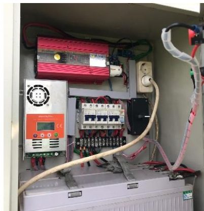
Figure 6. Water Tank Electric Control Box
