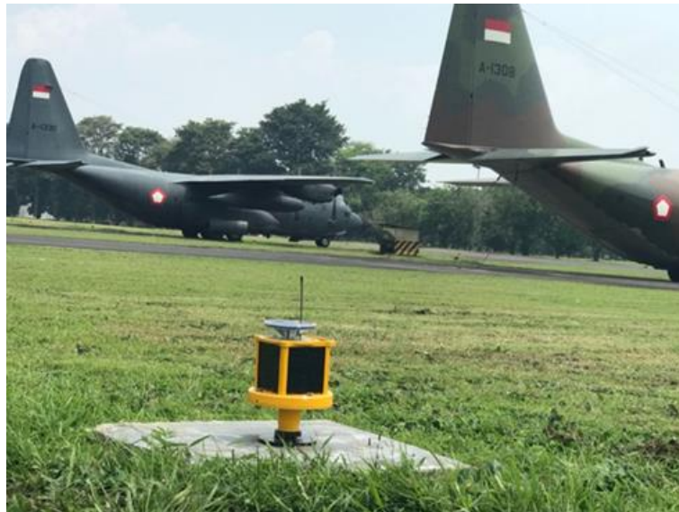
Figure 3. Solar-powered runway lights
